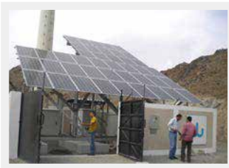
Outdoor Hybrid Base Station
